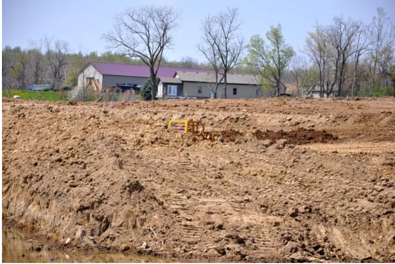
This picture shows the dozer down inside building one of the many surrounding ponds.
